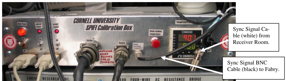
Figure 20: Sync signal cables on the electronic control box for the calibration unit.
