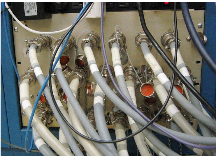
Figure 26. Front panel of the rack interface box.
