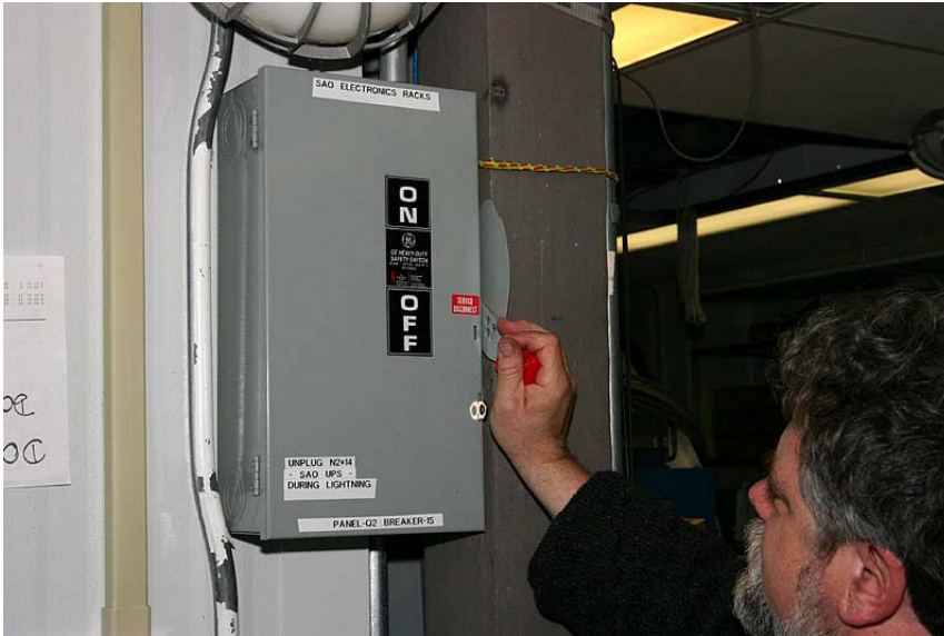
Figure 38. Main power switch.
