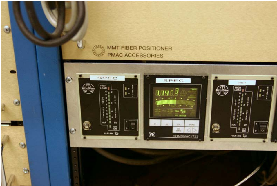
Figure 27. Hectospec ion pump is on the left, vacuum gauge is in the middle.
