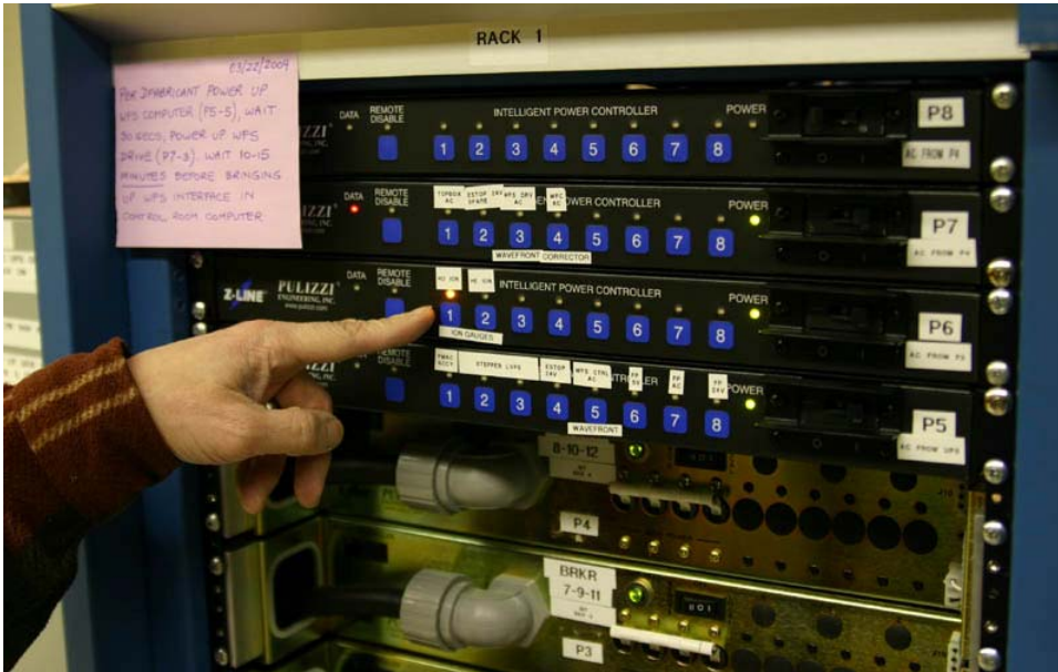
Figure 28. Power for the ion gauge. The main switch on P3 (gold-colored Pulizzi) must be on to power P6.
