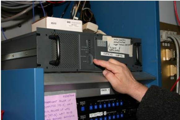
Figure 40. UPS on the top of rack 1. Rack numbering is from left to right.
