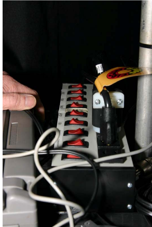
Figure 21. Power strip on pump station.
