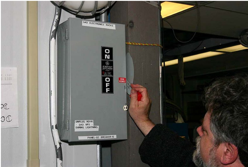
Figure 61. Main disconnect to the left of the electronics racks.
